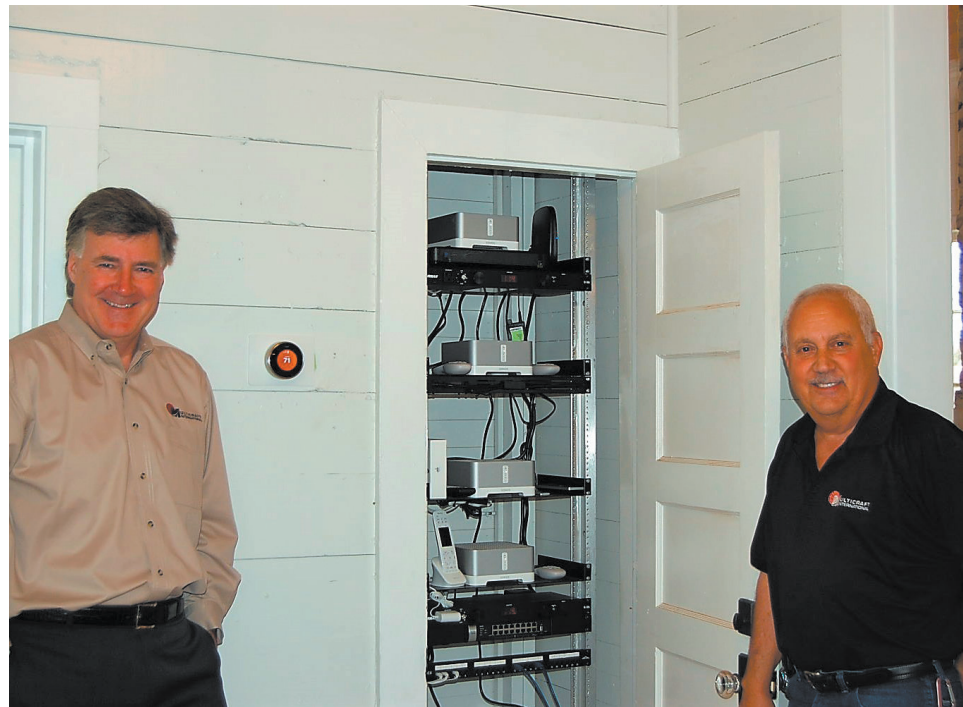
Andrew Mallinson, Multicraft CEO, left, is shown with Joe Ashker, Materials Manager, at the control center for the house's technology. (Photo by Susie A. Wolfe)
